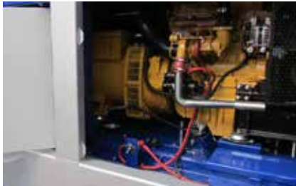
Diesel Genset - 87.5KVA LRC / 115KVA Tier 4 Final
